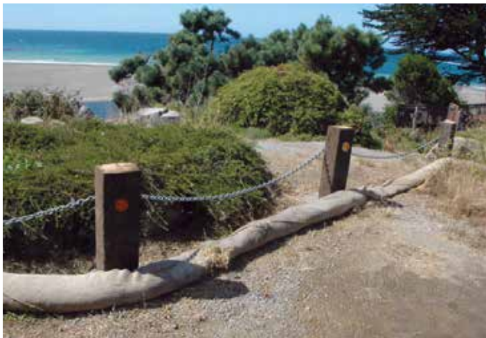
Replacing bollards that keep the trail separate from Surf Super's parking lot has become an important part of maintaining the Gualala Bluff trail. Twice during this past year RCLC has put in new bollards to replace ones that had been damaged. Photo by Bob Rutemoeller
